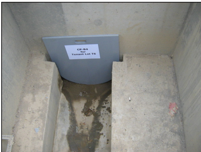
Figure 8-6 Stop-log in Place in Lot Occupied by Tenancy EP07-02
