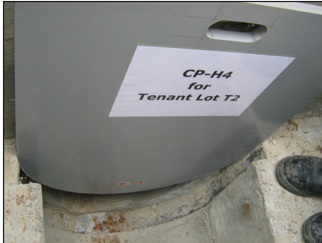
Figure 8-2 Stop-log in Place in Lot Occupied by Tenancy EP06-033 (1 of 2)
