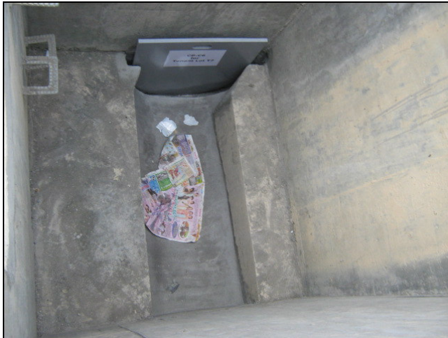
Figure 8-5 Stop-log in Place in Lot Occupied by Tenancy EP07-01
