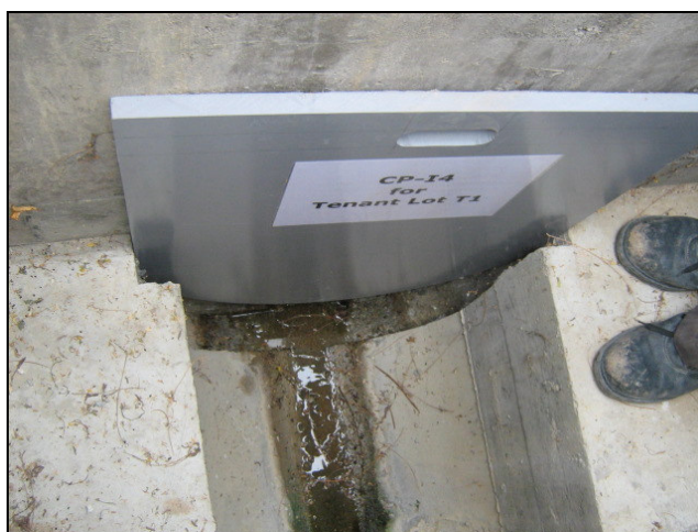
Figure 8-1 Stop-log in Place in Lot Occupied by Tenancy EP06-032
