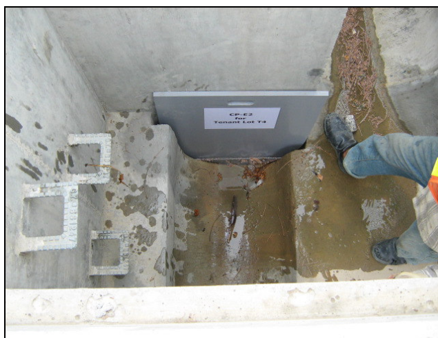
Figure 8-4 Stop-log in Place in Lot Occupied by Tenancy EP06-034
