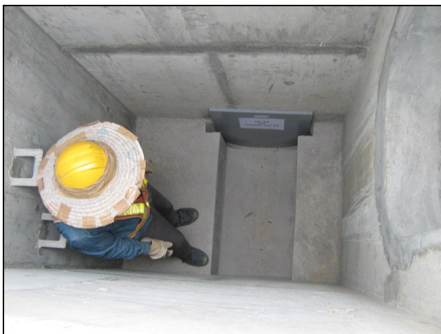
Figure 8-7 Stop-log in Place in Lot Occupied by Tenancy EP07-03
