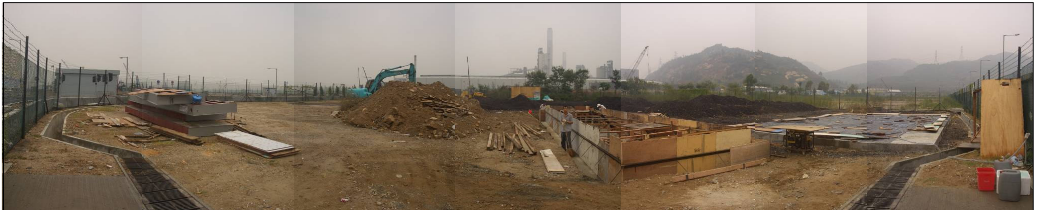
Figure 4-2 Preparatory Activities within Hong Kong Hung Wai Wooden Board Company's Lot (as of 31 October 2007)
